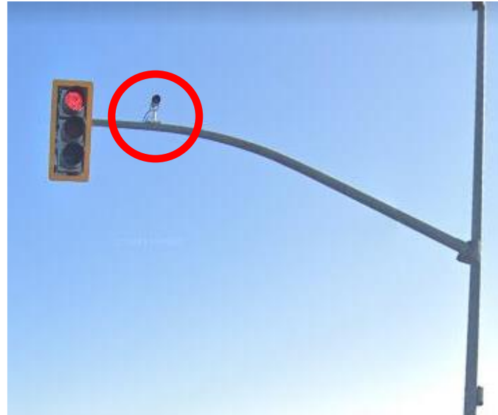
Fixed Intersection Camera (Closed-circuit television)
