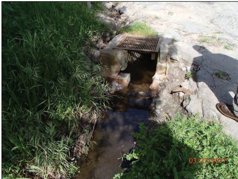
Photo 24 (Site #23): View of the outlet of the culvert at stream crossing Site #23 at the edge of the main parking lot. This culvert is undersized and stream flow avulses out of the drainage alignment and onto the parking lot surface.
