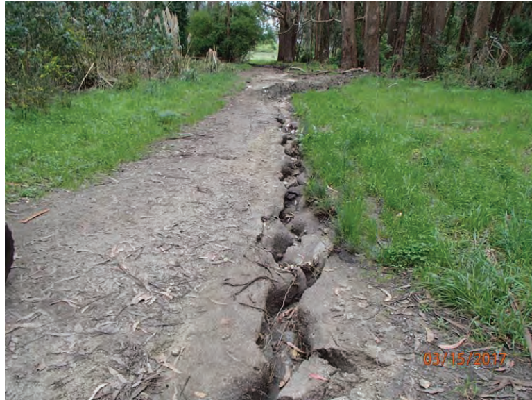
Photo 3 (Meadow Trail): View of active gully erosion along the Meadow trail. Combined diverted stream flow and concentrated road runoff are eroding the road surface along this native surfaced road.
