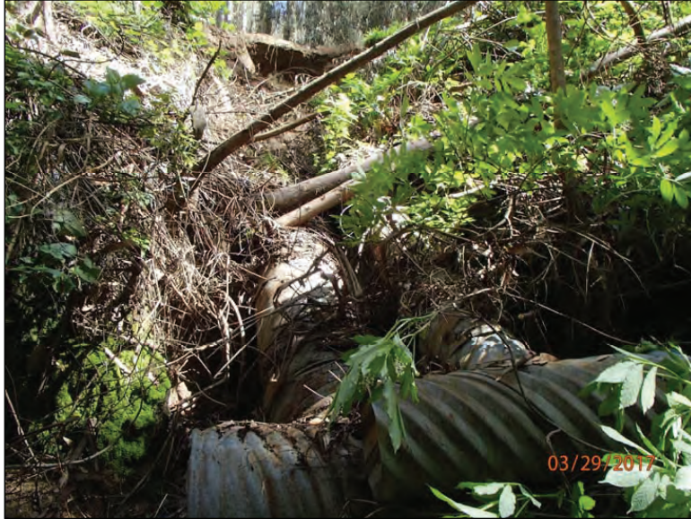
Photo 15 (Site #39): View looking upstream at the failing outboard fillslope of this plugged stream crossing. The photo was taken standing approximately 8ft downstream of the culvert outlets.
