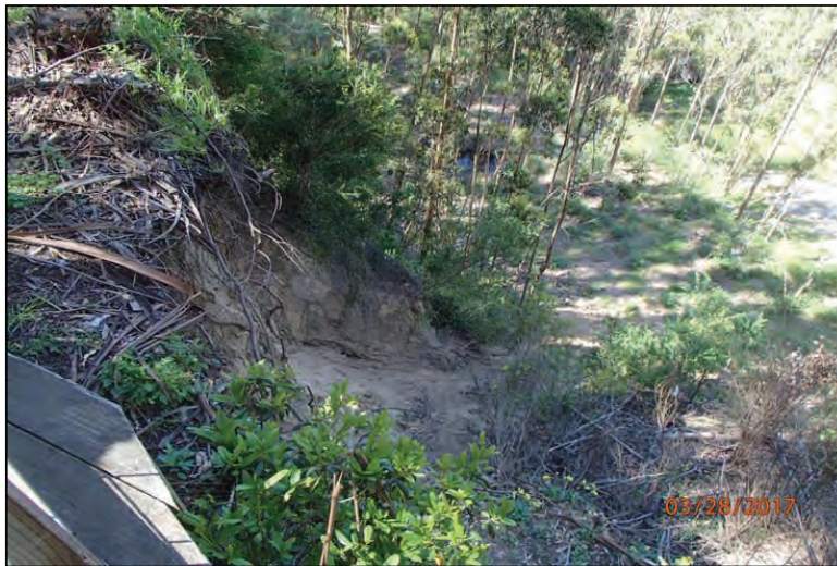
Photo 34 (Lookout Vista): View of the failing hillslope below the wooden lookout vista platform. The quarry cutslope is oversteep and is actively failing in multiple locations along the upper edge of the quarry area.
