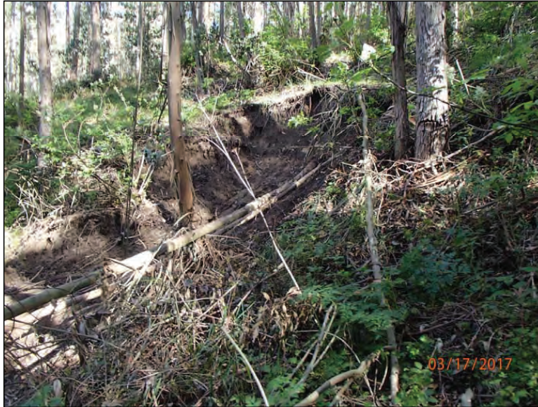
Photo 11 (Site #19): View of failing cutbank immediately upslope of the right edge of stream crossing Site #19. This cutbank failure delivers directly to the Class III stream in the axis of the crossing fill crossing.
