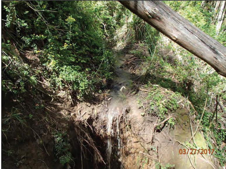
Photo 7 (Site #4): View of a road fill failure caused by diverted pond outflow. This erosion feature is located down the right road from the levee. Note the road prism is completely washed out.
