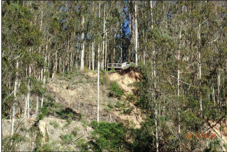
Photo 33 (Lookout Vista): View of the lookout deck and failing hillslope below the outermost footing. This photo was taken looking upslope from the base of the quarry floor.
