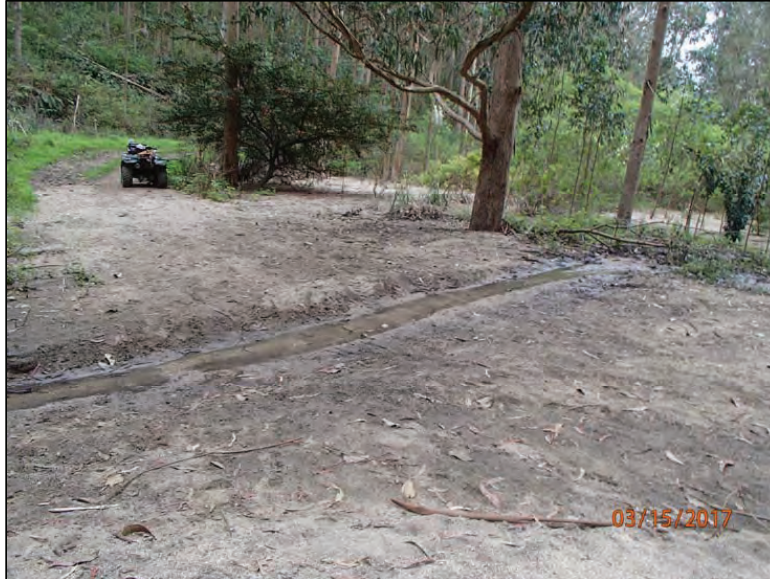
Photo 9 (Site #2): View of stream crossing through this shallow sediment filled pond. Stream sediment transport has deposited a large volume of fine sediment in this old pond, inundating the pond and trail.
