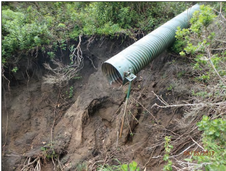
Photo 16 (Site #40): View of a section of disconnected culvert downspout at the top of an actively migrating headcut and gully below the paved Private Drive at Site #40. Oxidation exposed on the stake is indicative of the previous depth of burial prior to the episodic hillslope failure.
