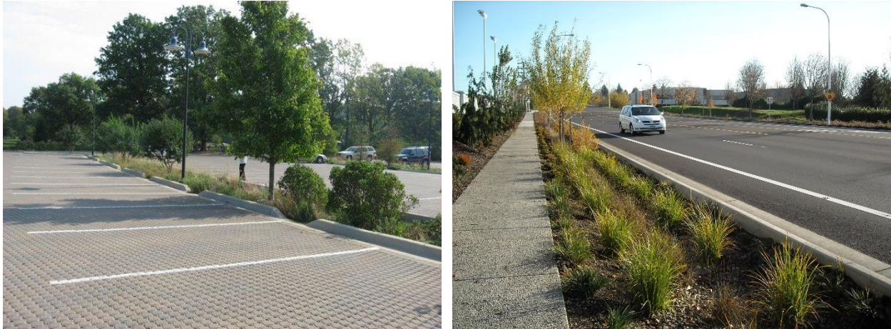
Figure 4-3. Example permeable pavers with bioretention cell at a parking lot (SMCWPPP 2009) and a vegetated swale along an arterial street (SMCWPPP 2009).
