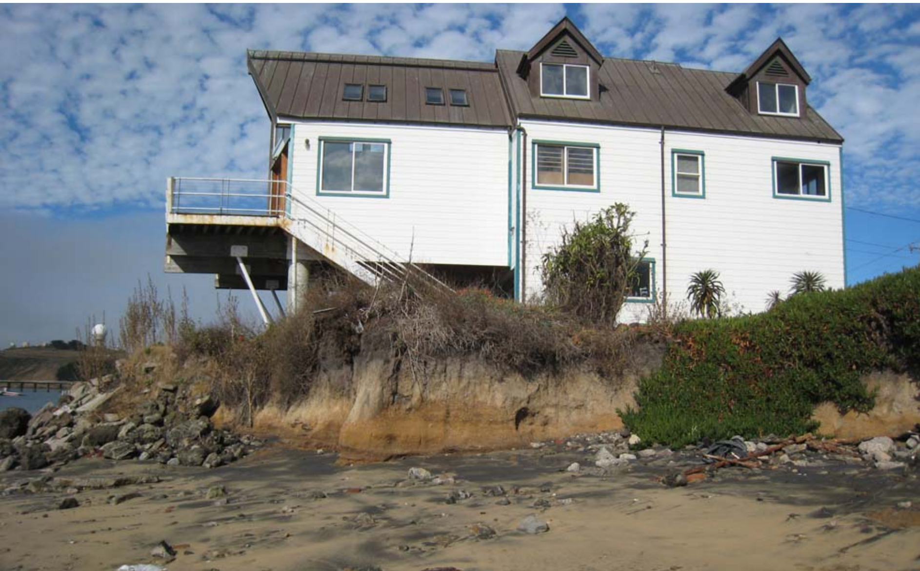
Extensive erosion of parcels next to riprap
